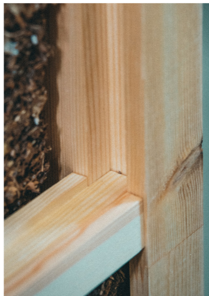
Inbetween the composite panels, struts are placed in the grooves to further stabilize the structure.
