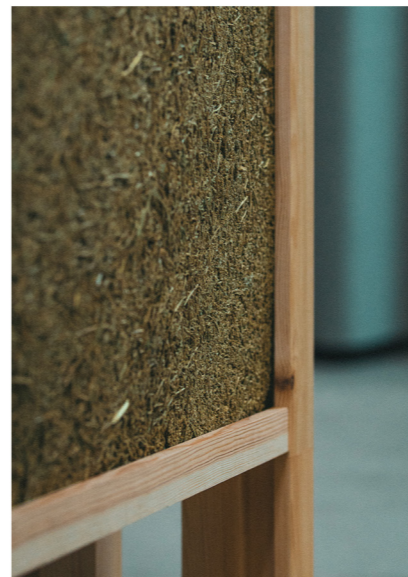
A view of the bottom interior composite panel (pine needles) it rests on top of a strut and inbetween the studs.
